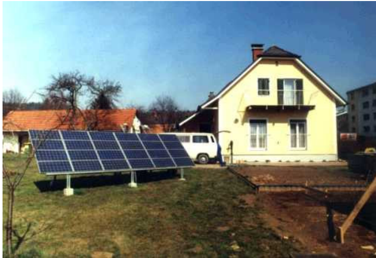
FIGURE 11: 750 Wp Solar PV Unit
