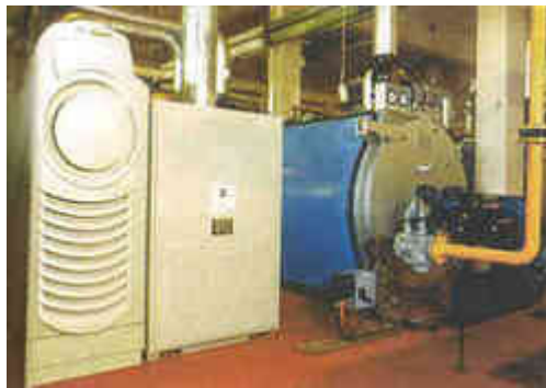
FIGURE 8: Capstone Microturbine - Generator System
